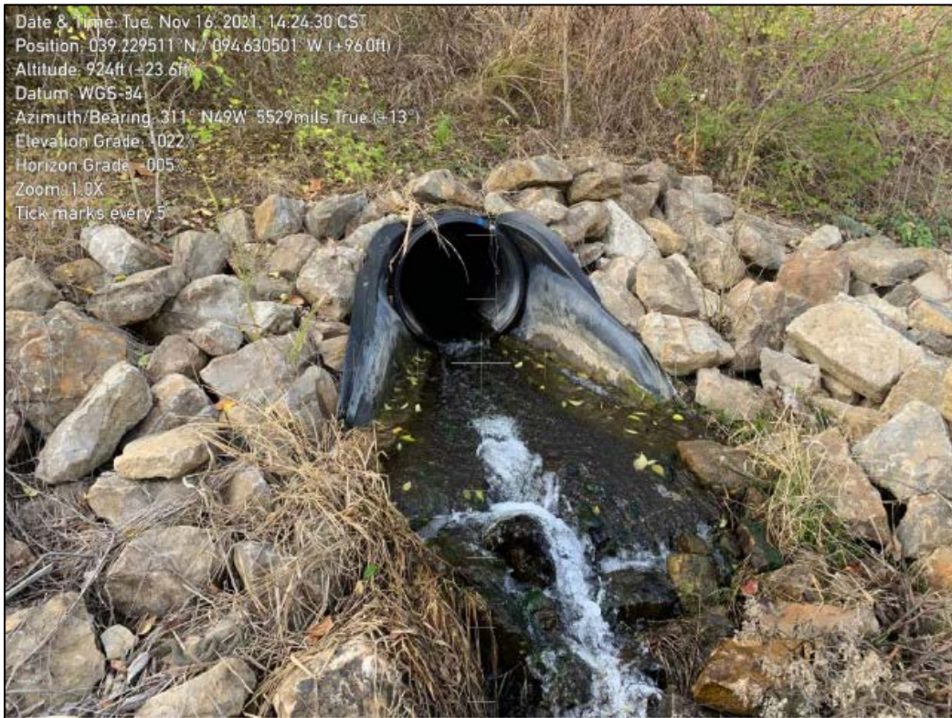
Figure 6- East Abutment Seepage Discharge from 24-in HDPE
