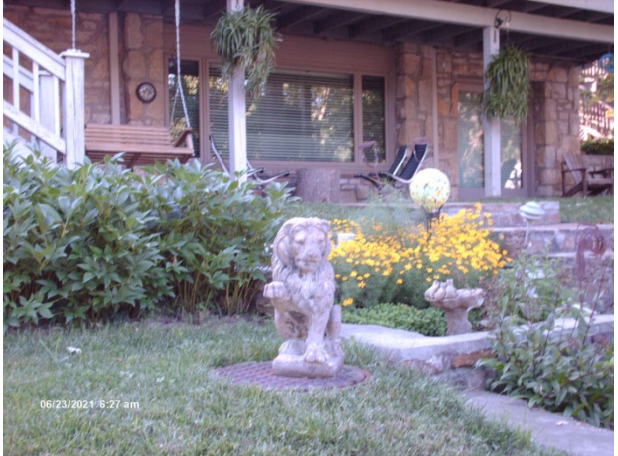
Manhole S09. Lid and statue are blown off from 900 Block Pump Station discharge, flows to lake.
