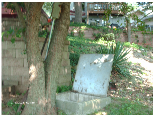
View of heaved MH, picture at left. Costly to replace due to wall and landscaping.
