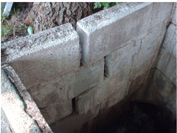
Rectangular block manhole badly heaved by adjacent retaining wall.
