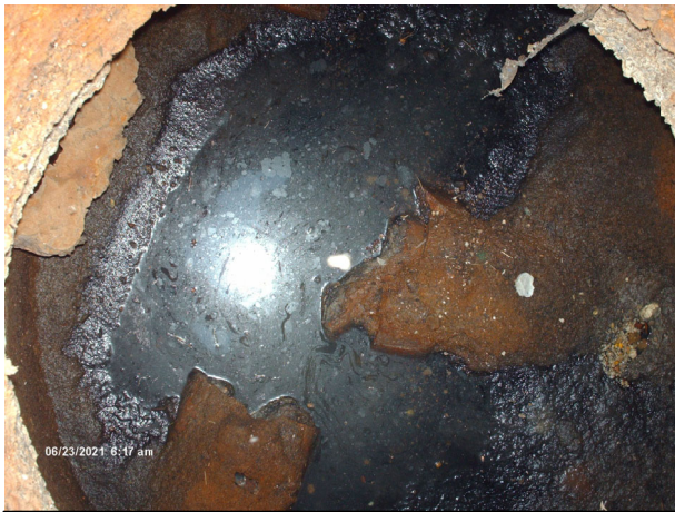
Pipe geometry poor, no bench, reduces capacity, creates back-ups.
