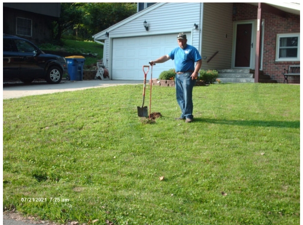
Manhole located, buried 18" deep in yard. City staff can raise to grade.
