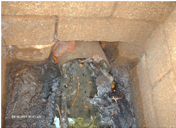
Rect. block manhole. Mortar is gone, holes allowing soil and water to enter.
