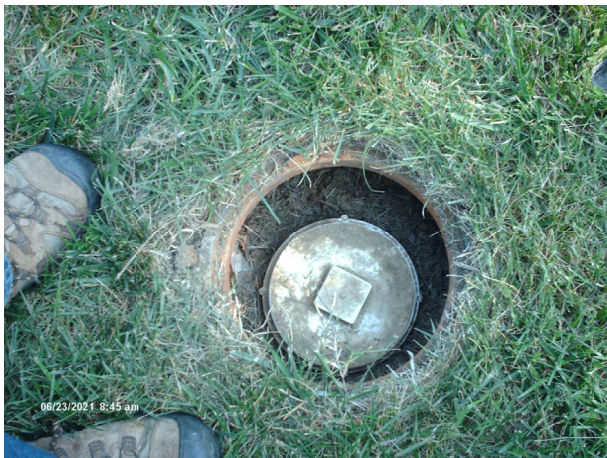
Small PVC cleanout on main sewer line. Need to replace with manhole.
