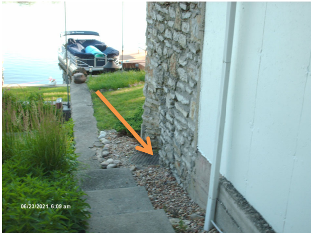
Masonry porch built over manhole. Nearly impossible to excavate here.
