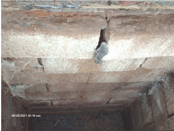
Typical rectangular block manhole. Mortar is gone and wall is heaved.
