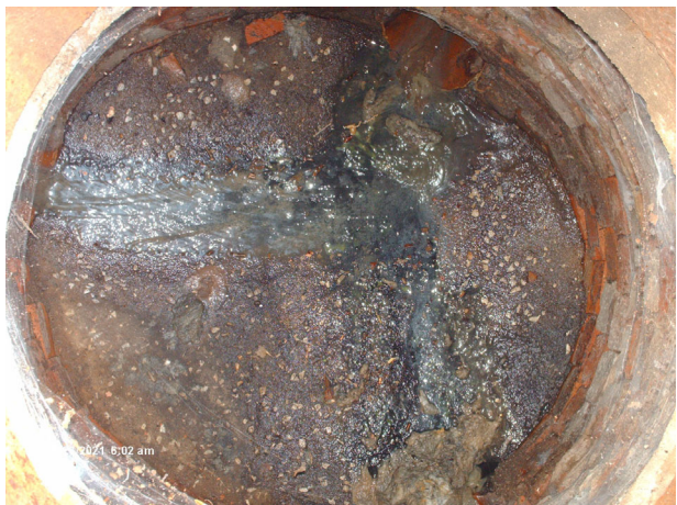
Brick manhole has no bench (channel in bottom). Causes debris to clog, and odors.
