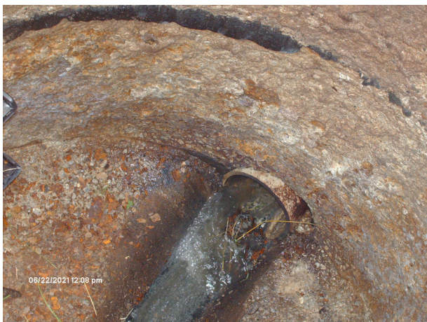
Newer pre-cast conc. Manhole, with MIC corrosion from H 2 S gas. About 1-inch gone.
