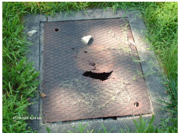
Rect. block manhole. Loose fitting lid, rusted through. Safety concern.
