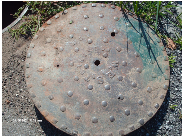
Some lids have vent holes, allow water inflow, this one in ponding area of intersection. Replace.
