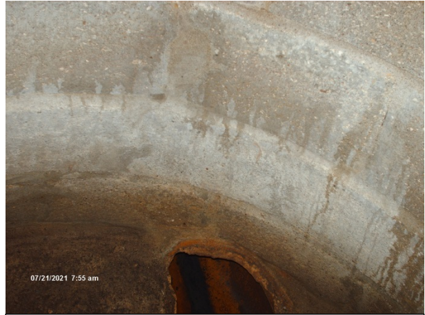
Typical round block manhole. Mortar is soft but wall is stable, can be rehabbed by lining.
